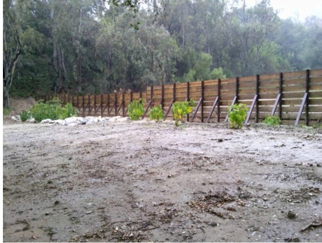
Figure 1. Photograph depicting rail and timber mudflow barrier
