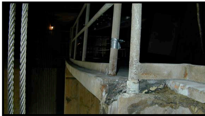
Figure 3. Existing slab deflection (measured at site visit as up to 2.5 inches)
