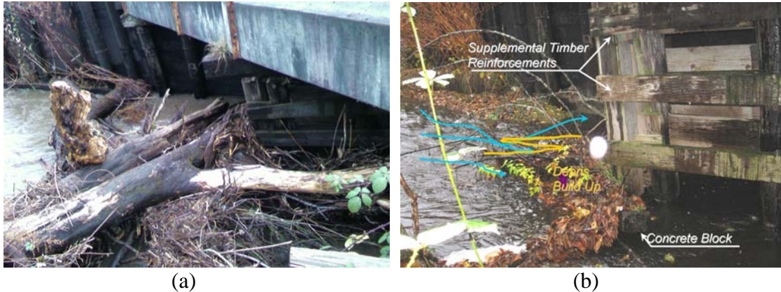
Figure 2. State of Center Pier, a) Condition after a Storm, b) Structural Retrofits
