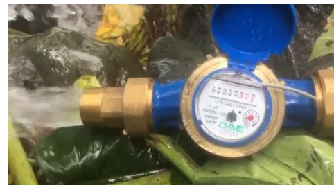
Figure 5: The new water system can provide 35-gpm of water to the community.
