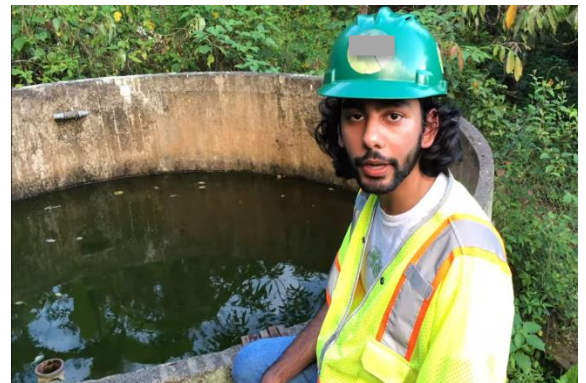
Figure 1: Nonfunctional Gravity Sand Filter
