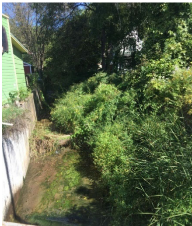
Figure 5: Existing conditions of vegetation overgrowth in the channel
