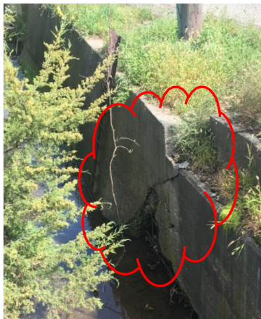
Figure 6: Existing conditions and deterioration in the channel
