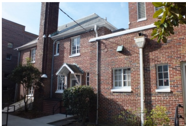
Figure 6. Back of church structure. Unbraced chimney near the exit is a life safety issue due to high seismicity which was not considered during original construction in 1939.
