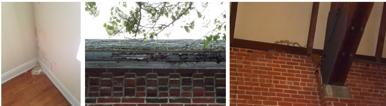
Figure 3. Examples of church deterioration, including peeling paint caused by excessive water on masonry (left) caused by leaky gutter (middle), as well as evidence of leaky roof (right).
