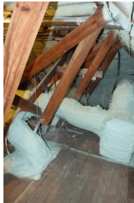
Figure 5. Wood brace cut for duct passage. Structural engineer made a quick calculation in front of the students and determined that the brace was redundant and not needed anyway.
