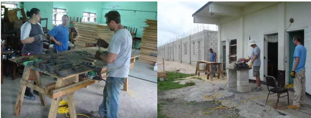
Above: (left) Students and faculty work together to fabricate the 700 stirrups required for the roof beams using ingenuity and a portable rebar bender and cutter. (right) Students, faculty, and village volunteers working together to prepare materials for the concrete roof.
