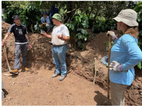
REIC explaining engineering concepts to the student team at the distribution tank site
