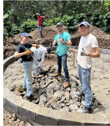
Rocks collected near the tank site were used for the tank foundation
