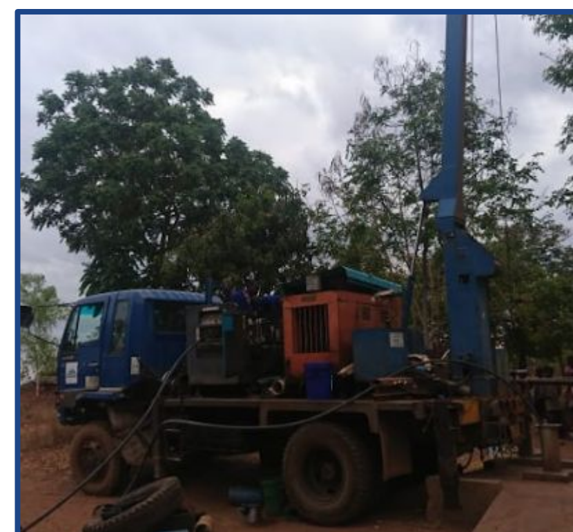
Pump test rig in the field
